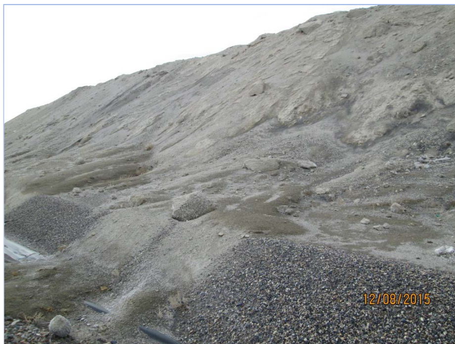
Photograph 0034: Localized sloughing of ash fill on east side of Cell 1.
