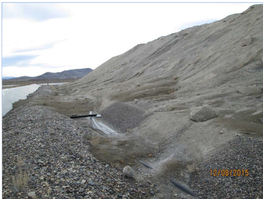
Photograph 0033: Localized slough on east side of Cell 1 (collection channel area).
